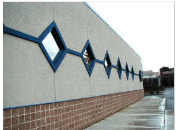
Inappropriate: Horizontal wall character exaggerated by the lack of wall definition and the oddly sized and shaped windows
