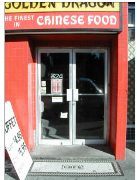
Inappropriate: Unpainted aluminum door frame
